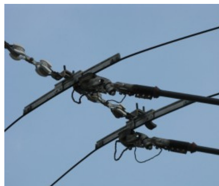
Overhead-contact with pantograph
